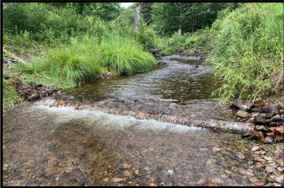
Digger Log installed in MacIsaac Brook, a tributary to the Ohio River
